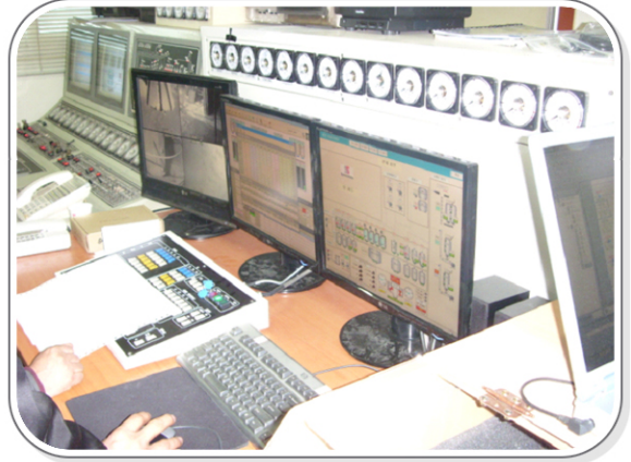
BP-210M3/HR CONTROL PANEL
