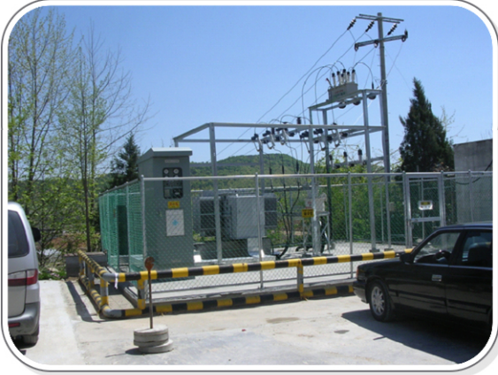
MAIN POWER ROOM-(SUBSTATION 650KW)
